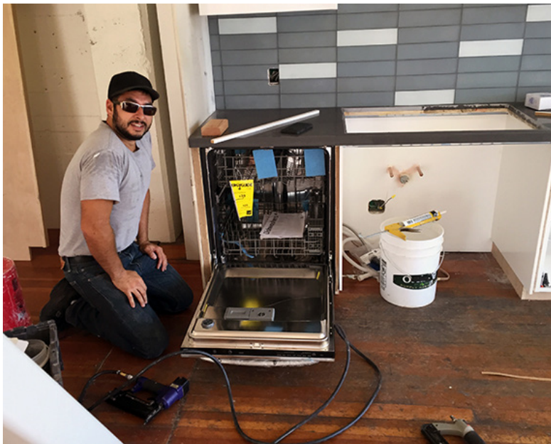
Conrad Meyers installs a new dishwasher in the new Root Division kitchen.
